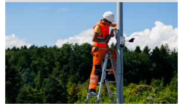
Installation and maintenance of sensors by qualified SWISSTRAFFIC staff.
